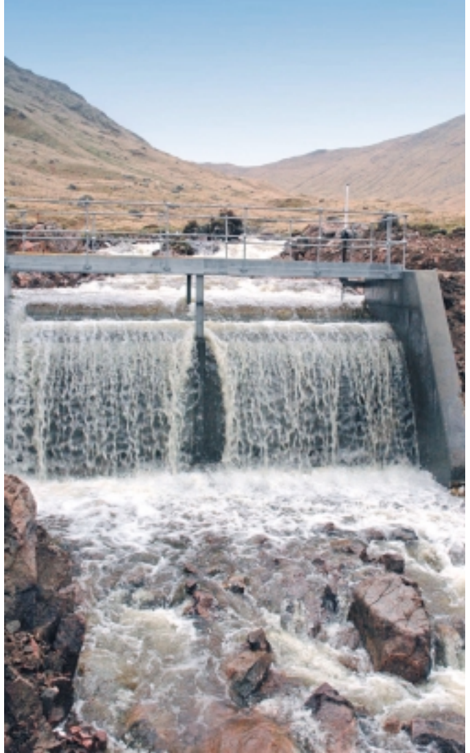
View of the Ghardail intake spillway, part of Scottish & Southern Energy's 3.5MW Kingairloch hydro scheme
